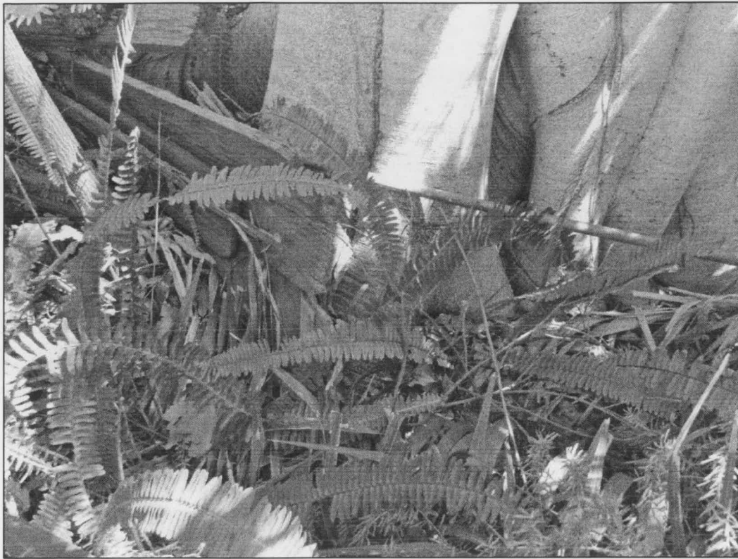
Figure 7 Showing root buttress of Tree 27 to the east, failed wooden fence in the foreground - only 1 root to the east which is supported by the root mapping
